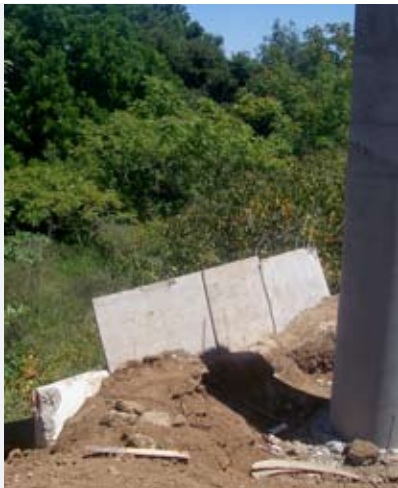
Figure 23. This barrier was placed to prevent sedimentation during road construction. Photo: S. Kocher.
