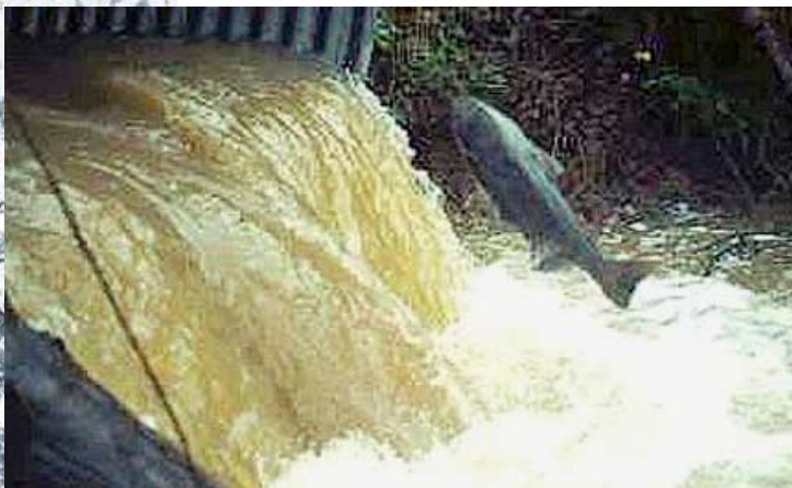
Figure 11. This culvert is a barrier to most fish that cannot make the jump into the culvert nor swim against the fast flow. Source: Courtesy FishXing, http://stream.fs.fed.us/fishxing/gbu/photos.html .
