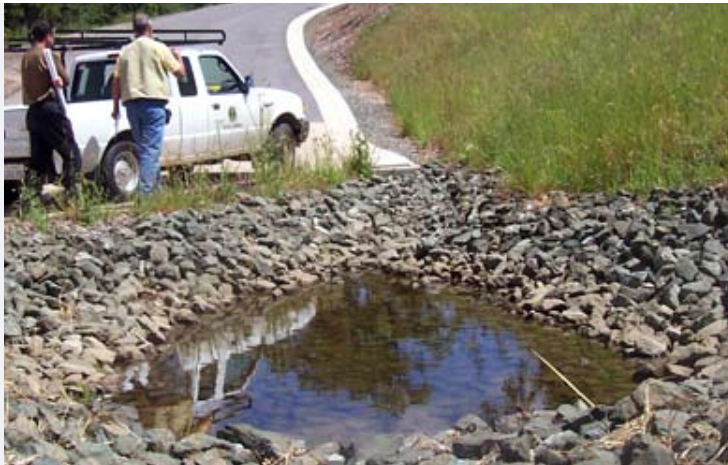
Figure 26. This detention basin captures flow coming off the road surface and ditch. It catches sediment and allows storm water to soak into the ground. Photo: S. Kocher.
