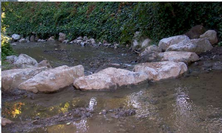
Figure 21. This rock weir has been installed to absorb the energy of the stream and reduce its ability to erode the banks. This helps reduce the need to install other bank-hardening measures that would impair aquatic habitat. Photo: R. Harris.
