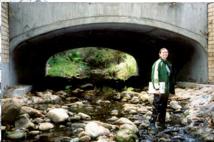
Figure 19. Prefabricated bridge crossing on a coastal stream in Ventura County, California. Photo: L. Thompson.
