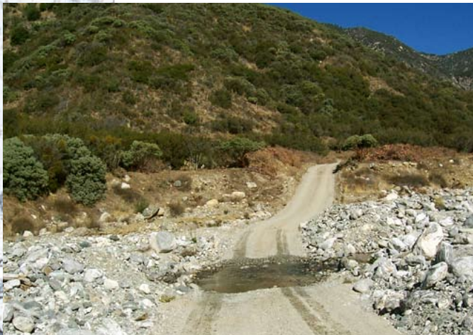
Figure 13. Low water crossings, also known as Arizona crossings, can pose a migration barrier to fish under certain flow conditions. Photo: R. Harris.
