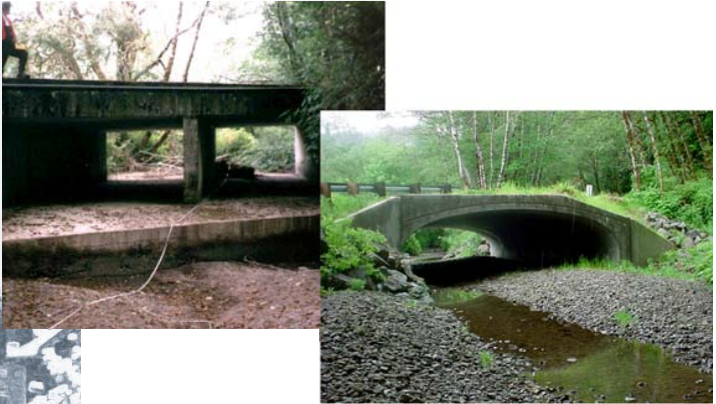
Figure 12. The double box culvert on the left was a complete barrier for all age classes of salmonids on Minot Creek in Northern California due to stream velocity, depth, and leap height. It was replaced by the bottomless concrete arch culvert on the right. The project opened up 2.5 miles of upstream habitat to salmonids. Source: Courtesy FishXing, http://www.stream.fs.fed.us/fishxing/case/ .
