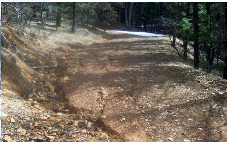
Figure 24. Erosion caused by ditch water leaving the ditch and traveling across the road. Photo: S. Kocher.
