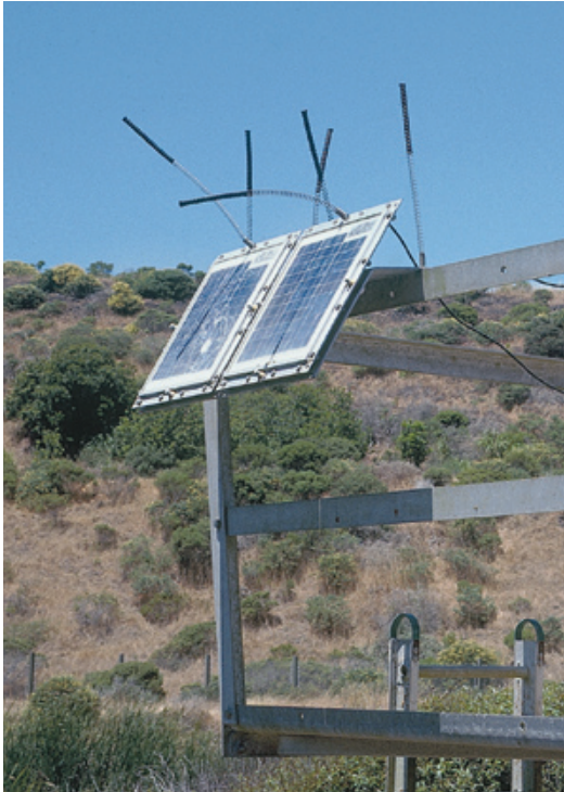
Figure 18. Springs and coils can be used as shown here on solar panels or on buoys or pilings to prevent perching. Photo: W. P. Gorenzel.
