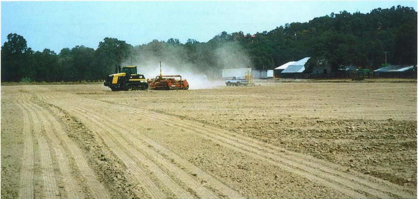
Photo 1. Land leveling to get the proper slope on a seedbed before planting.
