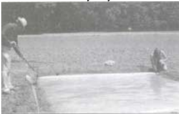
Figure 1. Applying clear 2 mil polyethylene tarps by hand Tarp is anchored to the soil by burying the edges.
