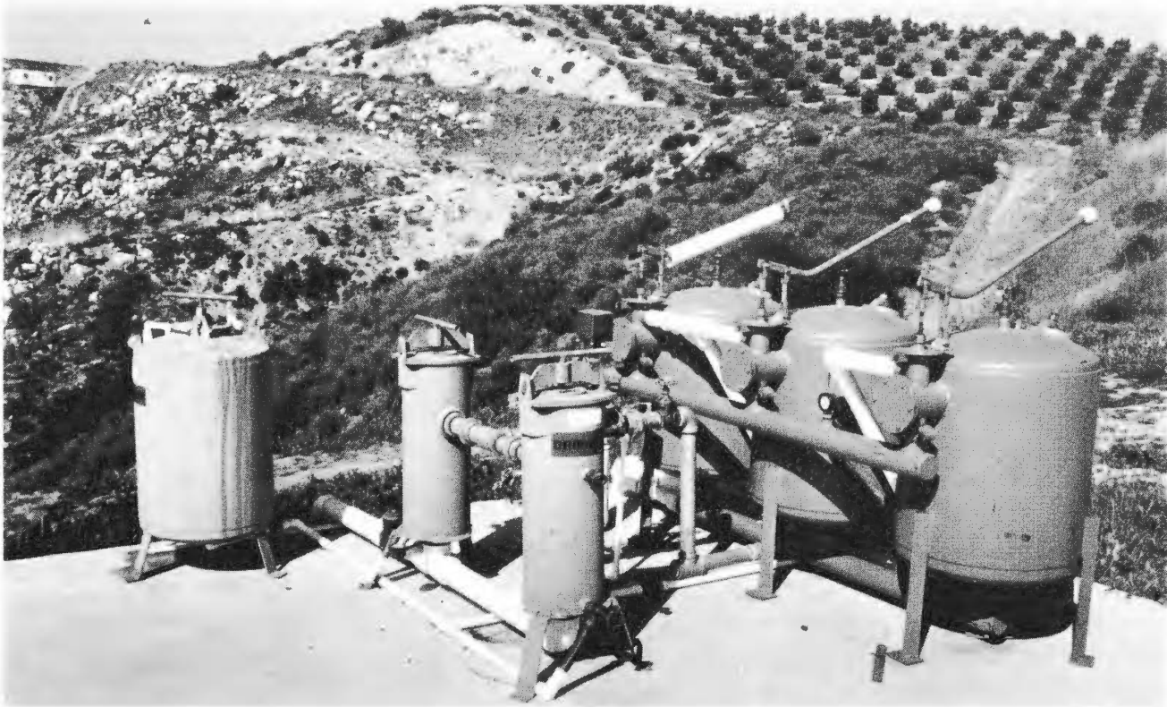
Typical drip irrigation control head.
