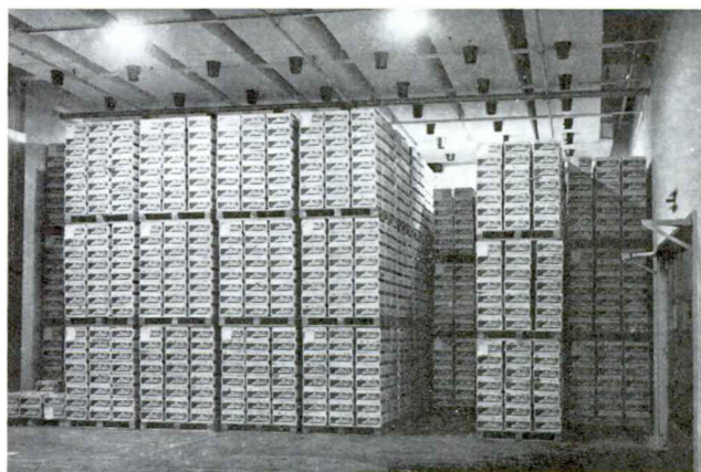
FIGURE 19. Cooling room with ceiling jets for air distribution.
